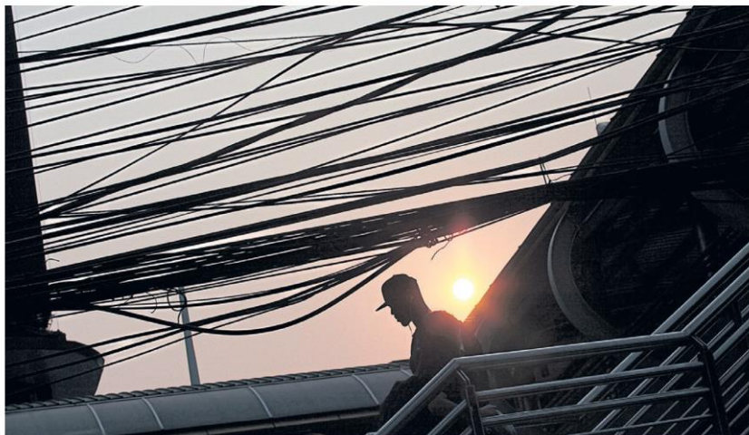
A man walks past tangled overhead electric wires at Bangkok's Sathon-Narathiwat intersection. PATIPAT JANTHONG
