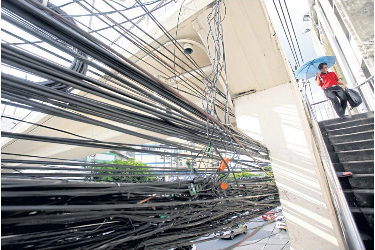
Telecom and cable lines along Phahon Yothin Road. The telecom regulator has ordered Krungthep Thanakom (KT) to renew its process of seeking operators to lease underground cable conduits. PATTARAPONG CHATPATTARASILL
