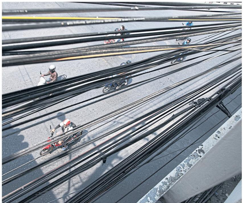
Motorcycles pass under overhead cables on Ratchadaphisek Road. TOT says conduits beneath 12 routes are ready to use. PATIPAT JANTHONG
