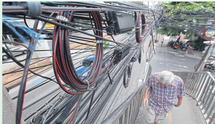
Communication lines and cables span electric poles on Phetkasem 48 in Bangkok. PAWAT LAUPAISARNTAKSIN
