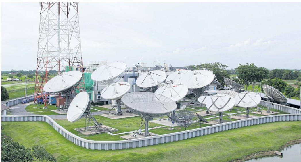
Satellite dishes at the Thaicom Teleport & Direct-to-Home Center in Pathum Thani.
