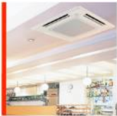
Air Conditioning Systems
