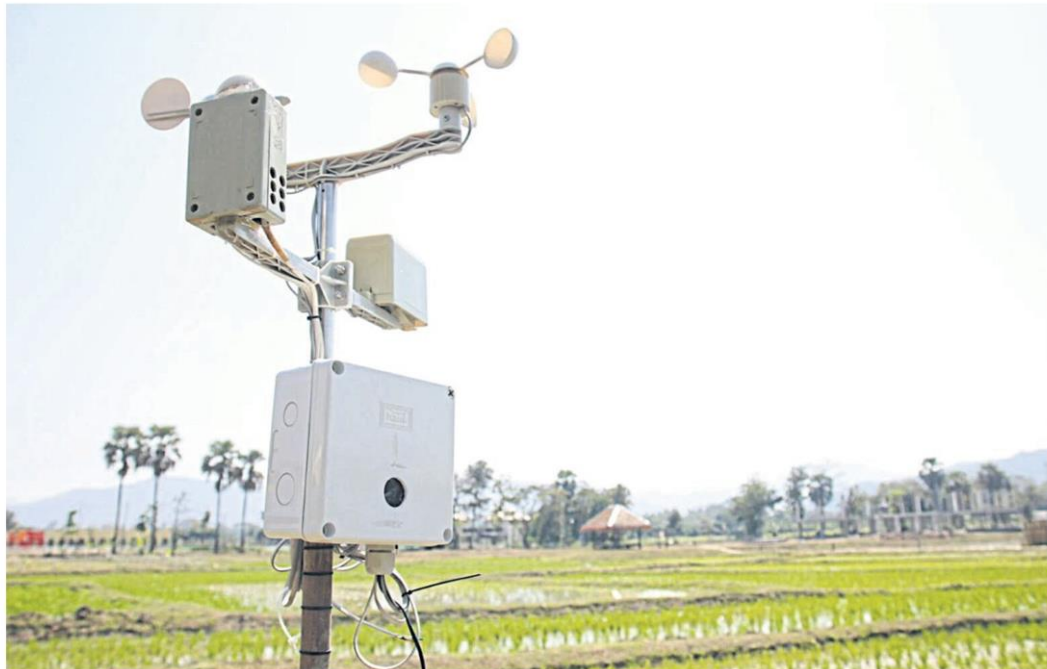
Communication equipment installed on the outskirts of Chiang Mai, which is intended to improve network access in remote areas.
