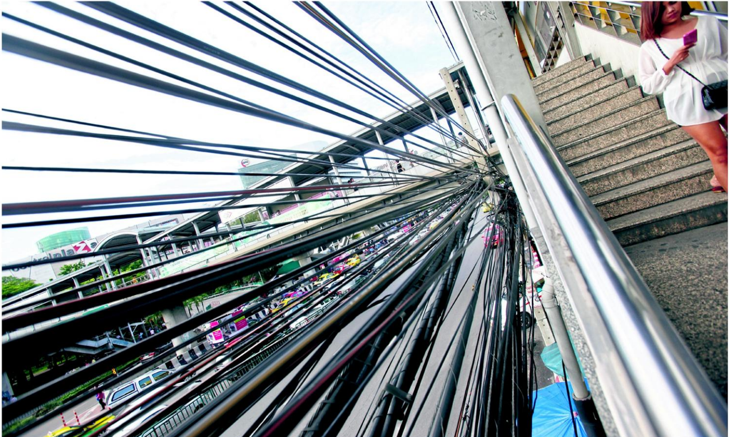
A woman walks past telecom and cable lines along Phahon Yothin road. The 4G auction is expected to spur huge investment in telecom lines. PATTARAPONG CHATPATTARASIL
