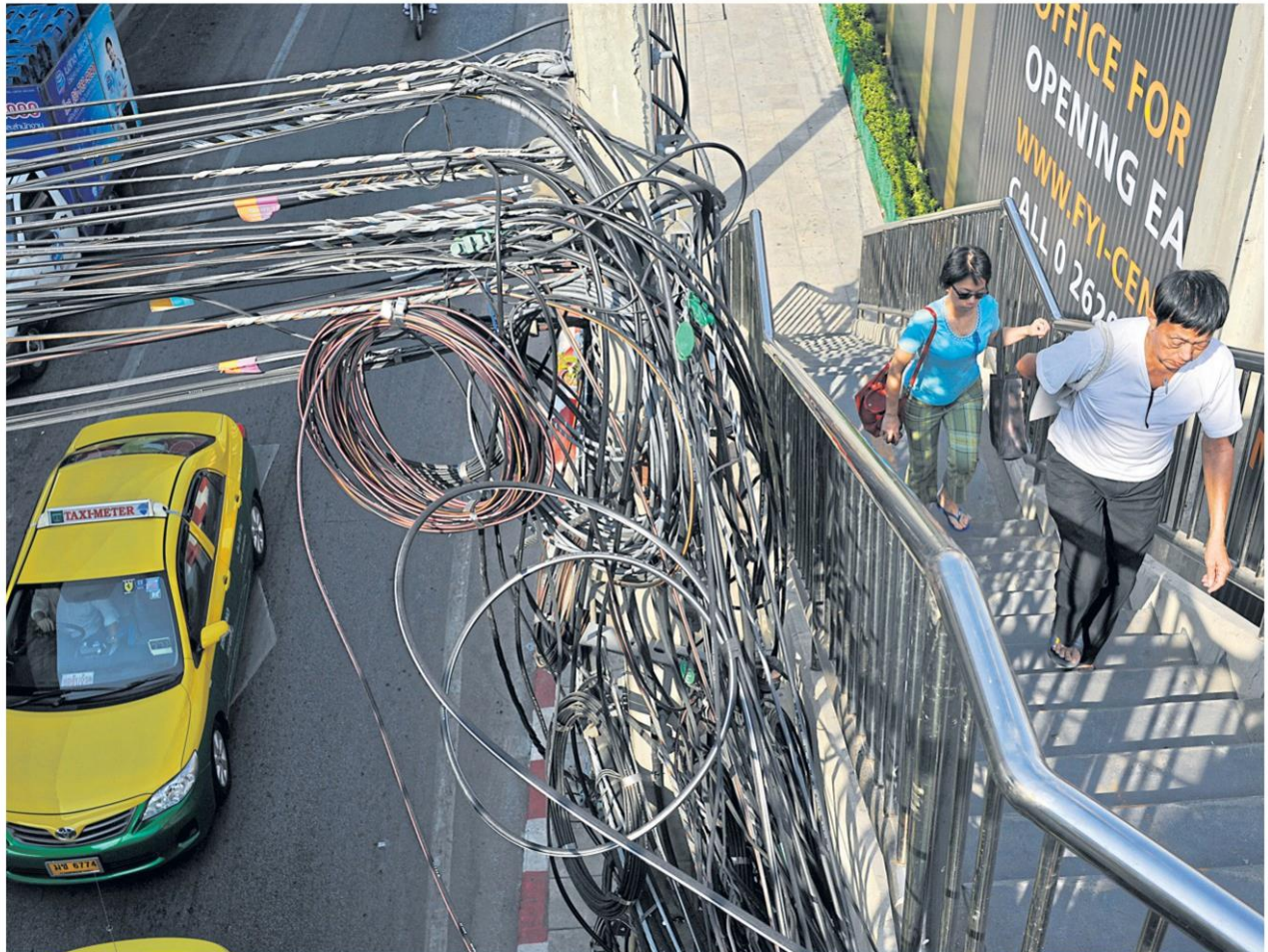
Wires are jumbled around an electricity pole next to an overpass at Ratchadaphisek junction. WICHAN CHAROENKIARTPAKUN
