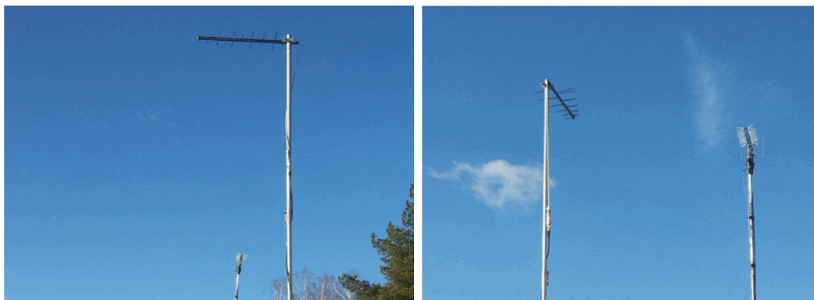
FIGURES 9, 10 Positions of TV broadcasting receive antenna and fixed wireless broadband access system transmit antenna
