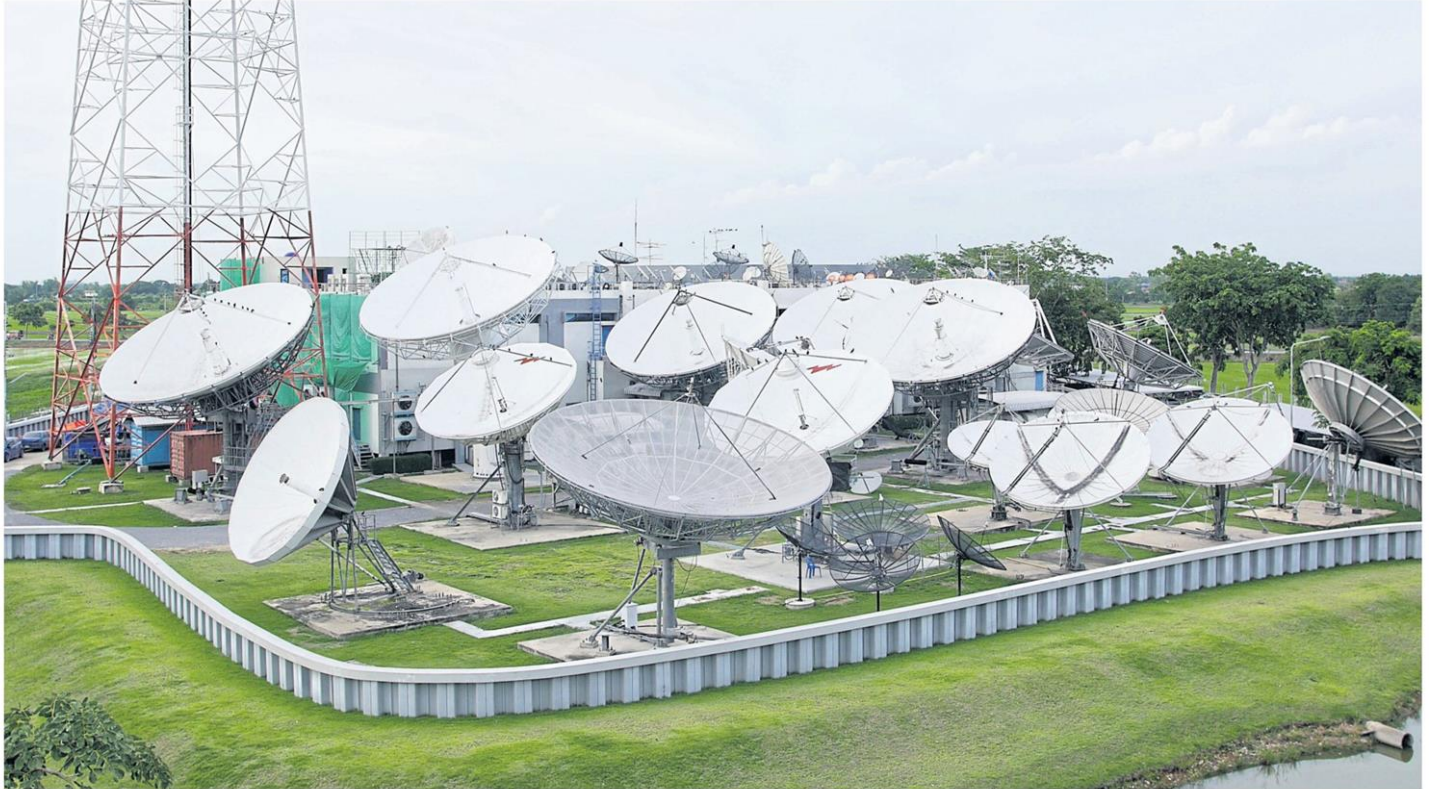
Satellite dishes at Thaicom Teleport & DTH Center in Pathum Thani province.
