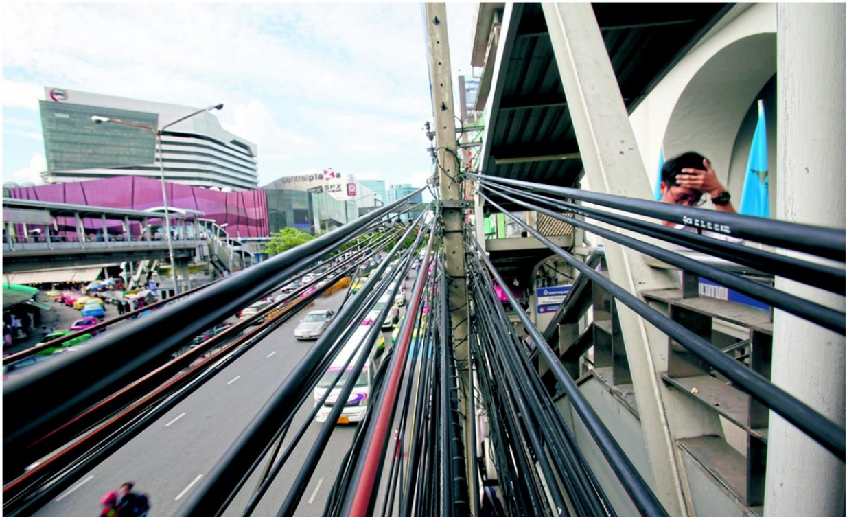
A pedestrian walks past a tangle of telecommunications and broadcasting cables on Phahon Yothin Road. CAT is considering allowing cable TV operators to use its fibre-optic network for free. PATTARAPONG CHATPATTARASILL
